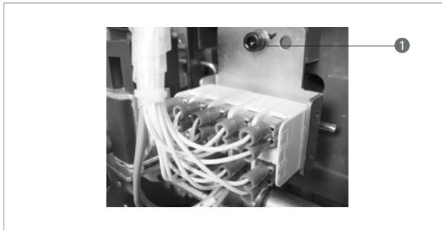
Fig. 14. Aux. switch general view
